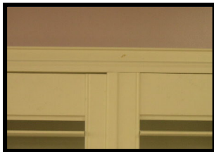
Once you have installed the panels, and they do not line up,
